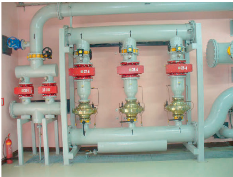
Gas drainage equipment at Pniówek Mine in Poland
